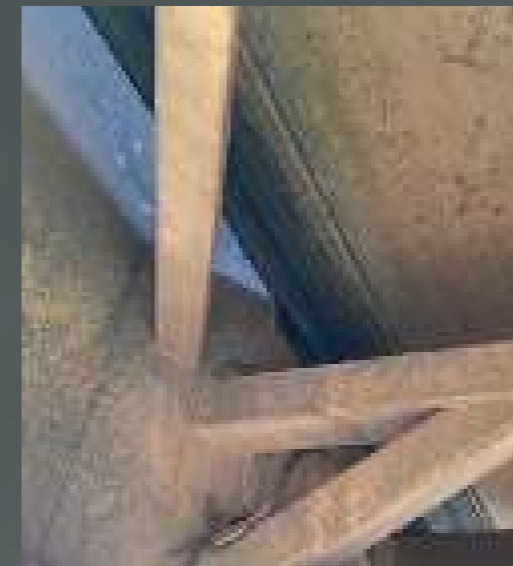
Conveyor belt already cutting into the supporting structure
