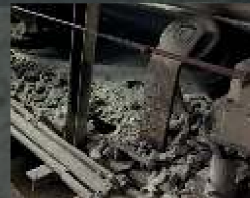
Soiling caused by poorly sealed transfer points
